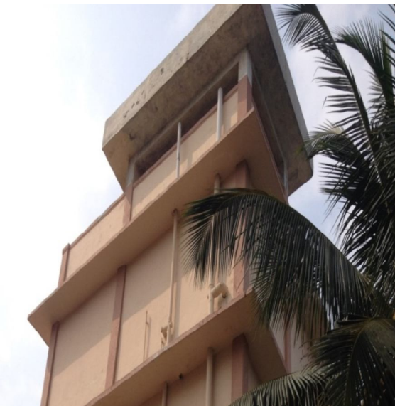
Fig 5.3b Vent should be 152m above the roof and it should not be near to any water source Ref:UPC2008 class 906.1
