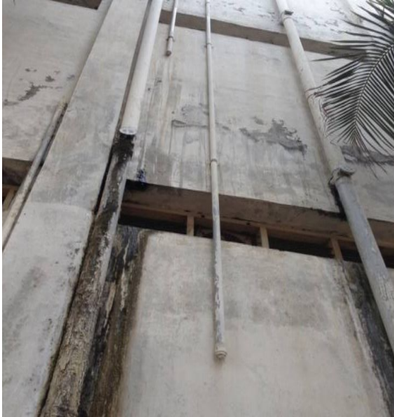
Fig 5.3.a Damage of walls due to absence of clamping
