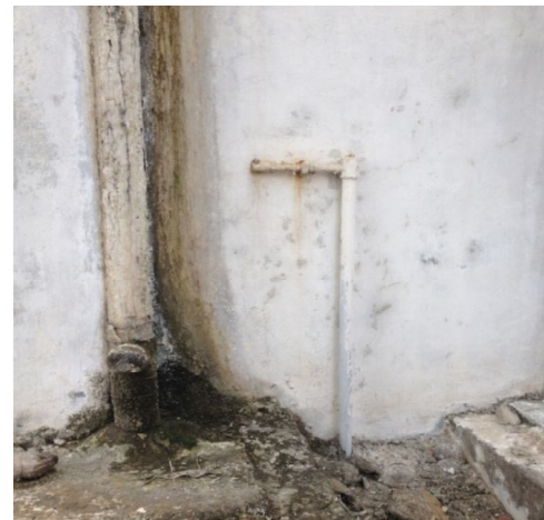
Fig 5.1 Clamping was not provided which lead to damage of Wall
